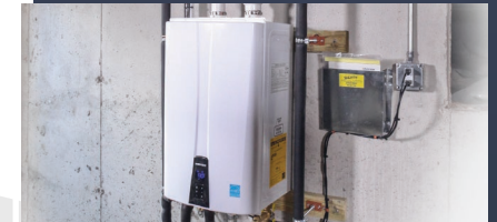
Plumbing & Water Heaters
